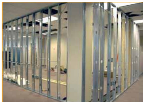
Also under construction is state-of-the-art Videoconference Center on second floor, progressing toward an autumn completion.
