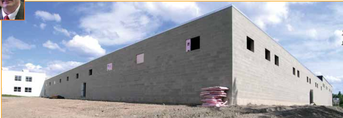
"New meets old" as the addition joins to our current side wall at left. (Lower windows look into Engineering; upper windows are USA Customer Service.) Addition wall at center faces Sheridan Drive.
