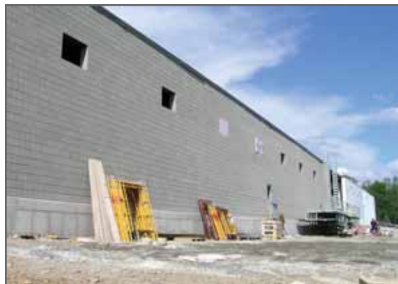
View from rear of building, joining our current warehouse (far right) with the new warehouse addition.
