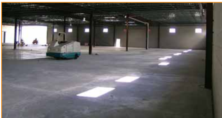
Future floor space of the Machine Shop. Area at rear left will house new Random Orbital Sander cell, with Stationary Machines cell next door.
